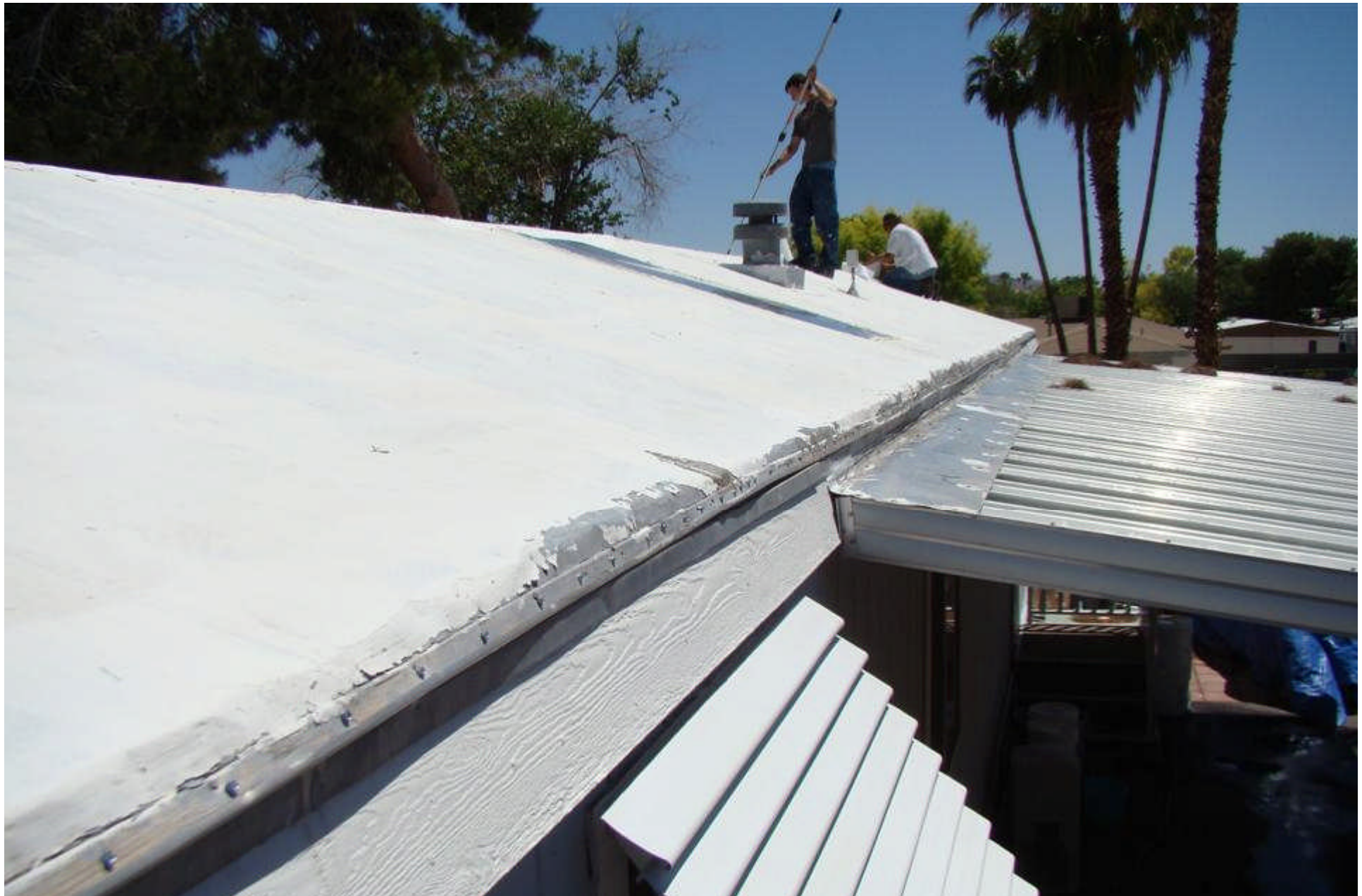
Kay's home in Las Vegas is getting a new Thermo-shield Roof. A Solar Difference, a local roofing contractor was chosen to do the installation.
